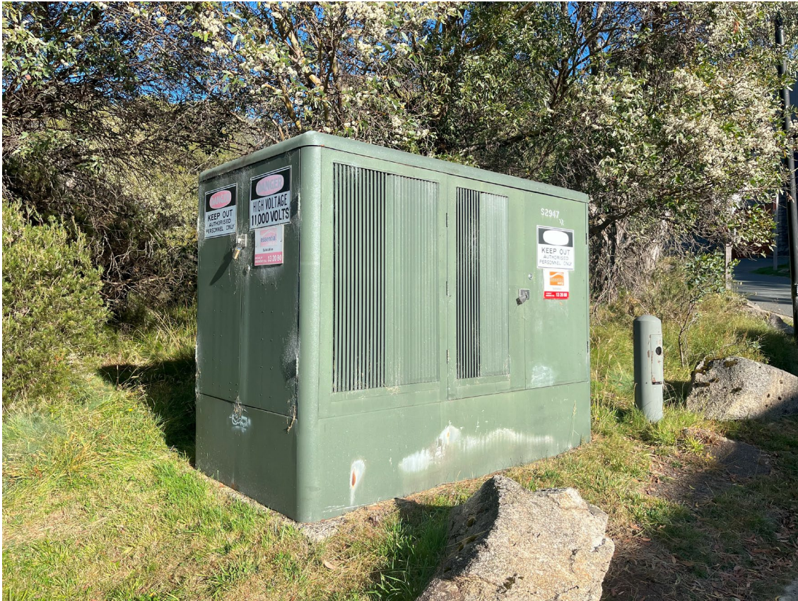
Figure 13: Example of pad mount substation
